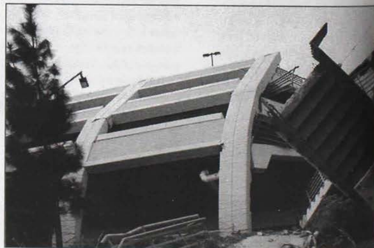
A collapsed parking structure on the campus of California State University in Northridge, home of Iota Upsilon Chapter.
