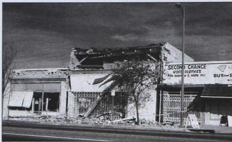
Businesses on Sherman Oaks Street in the Northridge area suffered major damage.
