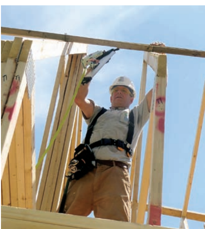
In Addison, Vermont, Gilmore's 24 th state, he sets roof trusses. "One of the wonderful things about Habitat for Humanity is it teaches volunteers a variety of carpentry skills and helps them to learn new crafts," says Gilmore.
