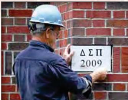
Stone Mason Walt Long puts the cornerstone in place, his last act before retiring after a long career, most recently with CR&R Construction.
