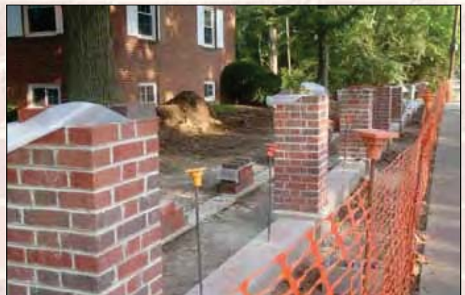
A new brick and wrought iron fence will line the Central Office along Campus Avenue.
