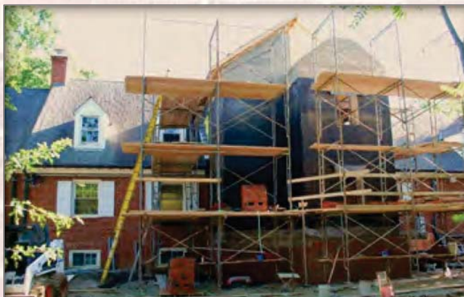
Final roof attachment for the new elevator/restroom tower took place in early September.
